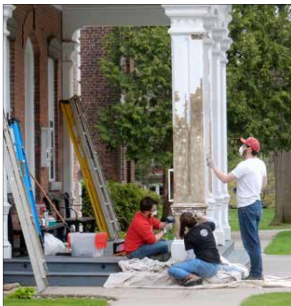
Old, peeling paint had to be scraped off the columns, railings and porches, before a new coat could be applied. The Mansion House has over a dozen porches, so this was no small feat!
