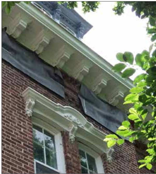
In July 2019, rubber sheeting was installed over the damaged areas of the Quad to prevent continued deterioration.
