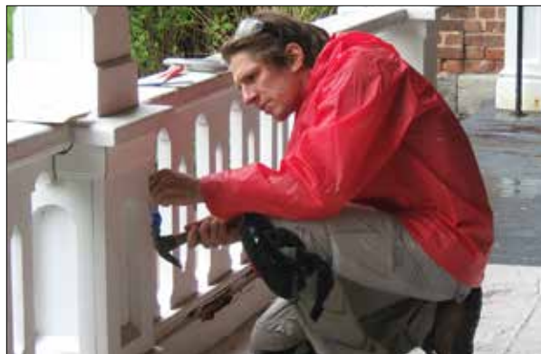
Sections of railing in need of repair or replacement were carefully deconstructed so as not to damage any sound historic material.
