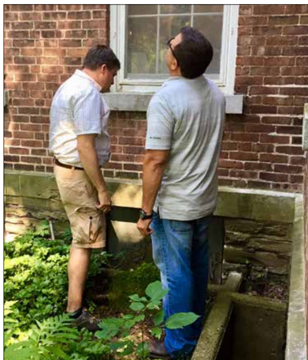
Jamie Trevvett and Scott Lupini, historic masonry expert and Vice President of Lupini Construction, examining the masonry on the Quad, below the damaged cornice line.
