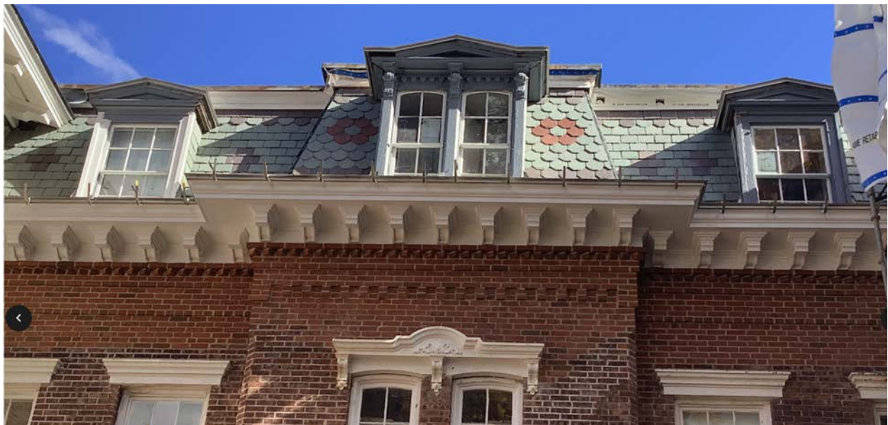
New slate, rehabilitated cornice and brick facade, West wall of the South Wing – 3/22-3/23
