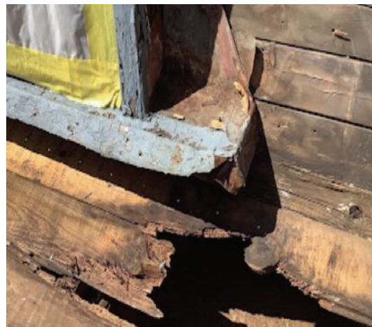
Before: Patched and leaking tin flashing, deteriorated wood cornice shelf & windowsill
