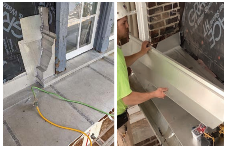
After: New Freedom Gray copper covered dormer tops. Shown is arched top & pedimented style – 6/22-3/23 New copper covered decorative bracket and mansard flashing
