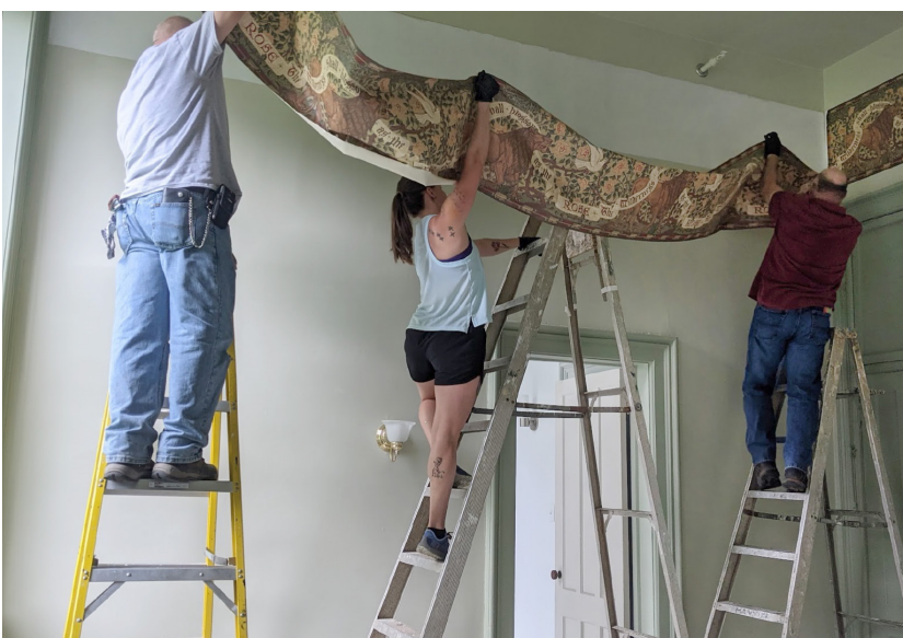
Left to Right: Jim Anderson, Chelsea Scheuerman, and Mike Colmey installing Bradbury & Bradbury's Lion and Dove frieze wallpaper in room 144
