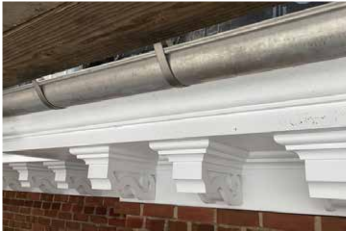
Installation of gutters to address water mitigation which contributes to wood rot and infiltration (Preservation)
