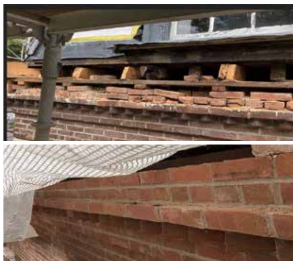
Replacing section of masonry wall and cornice which was too deteriorated for repair. South Wing, South Elevation, left of South Tower (Rehabilitation)
